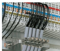
U-shaped (10 x 3) mm copper busbar
