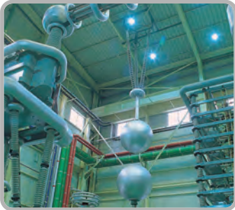
High Voltage Test / Impulse Test
